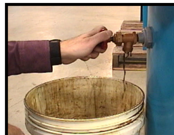
Purge oil into container .
